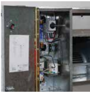
Starters and disconnects
